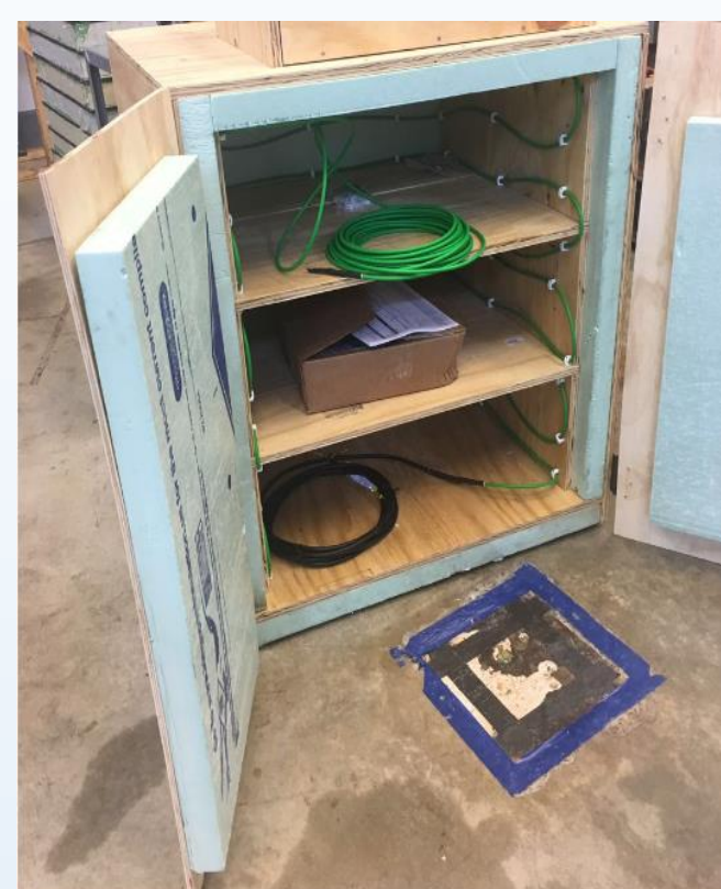
Box with heating system - 35°F
