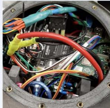
Fig 2. Internal wiring. VESC, Arduino, and R-Pi above batteries and motors
