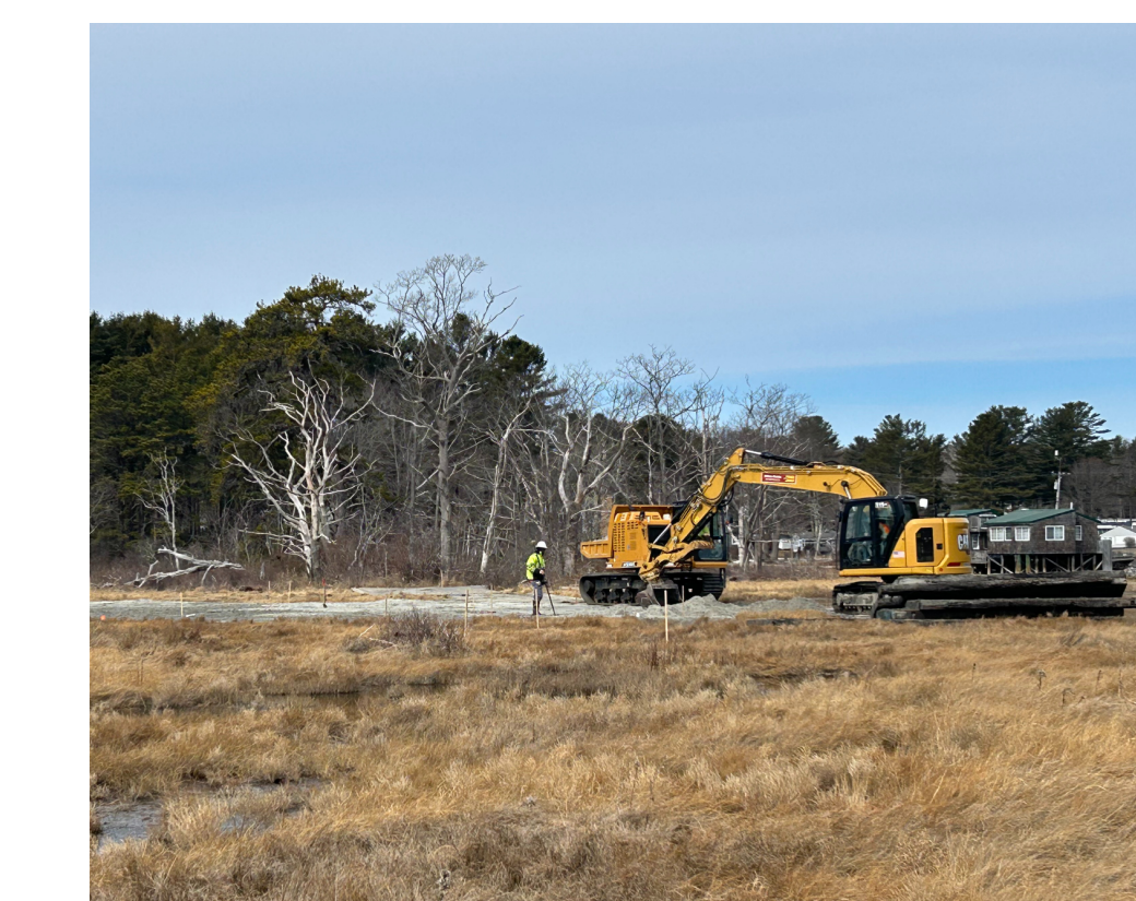
Figure 8: Sediment addition via thin layer placement at a marsh in Wells, ME.
